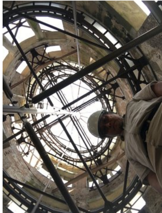
The recording takes 17 minutes, during which time the crew must remain silent. Earlier that year, the City had installed steel reinforcement to secure the dome interior. Courtesy of Alan Nakagawa.
